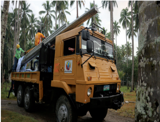
SOCOTECO workers start the energization of sitios in Barangay Datal Bukay, Municipality of Glan Sarangani
