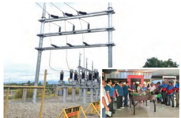
The 10-MVA substation and 69 kV subtransmission line located in Tubod, Lanao del Norte
